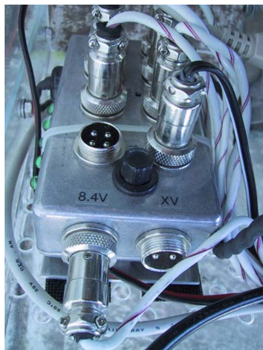
Figure 7-7 Power supply breakout box, with +5V, +9V, and +12V at each connector
